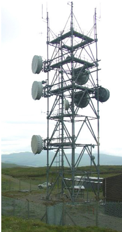
Figure 6a. Microwave repeater showing multiple co-located antennas.[3]
